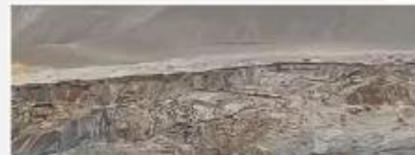
Reservoirs, at least 100 meters below the top of the tailings dam, were completely destroyed.
