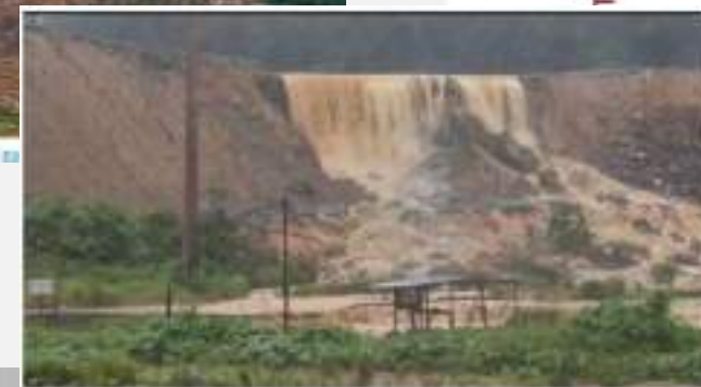
Major reportedly failed tailings dam at Bukit Mantri Gold Mine in Malaysia
