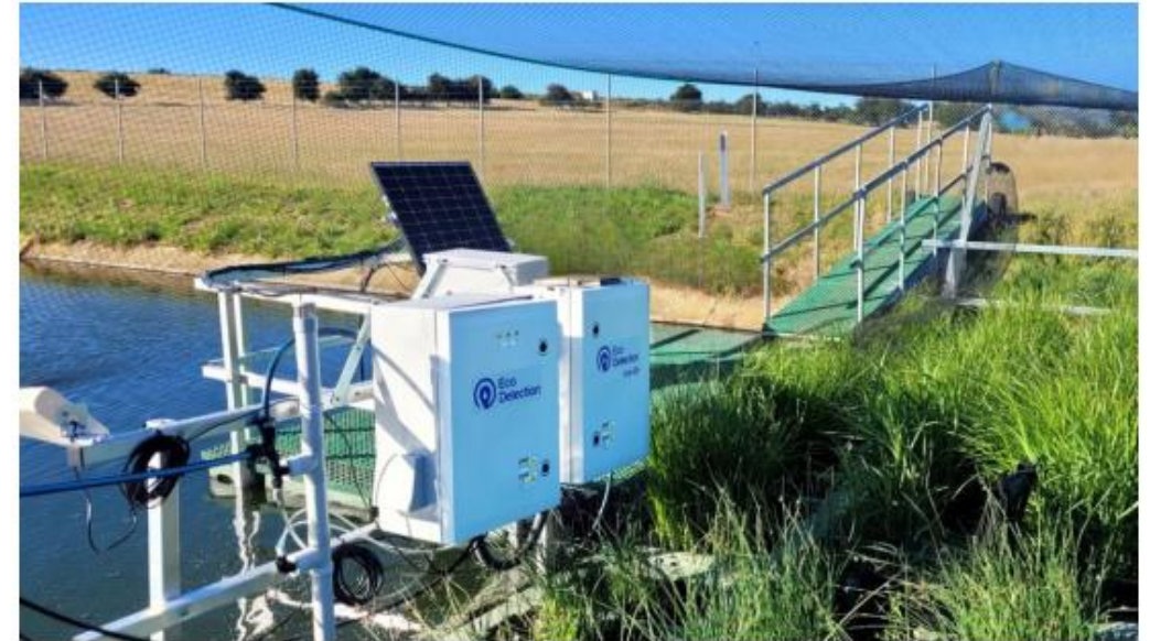
Ion-Q+ Installation at Western Junction Wetlands, Tasmania Australia.
